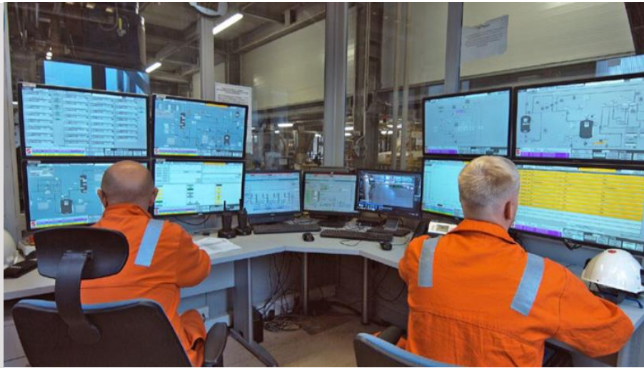
Central control room of Stepan Poland plant
